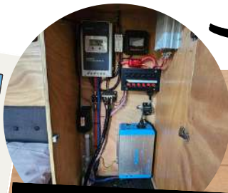
Off-Grid Solar System
